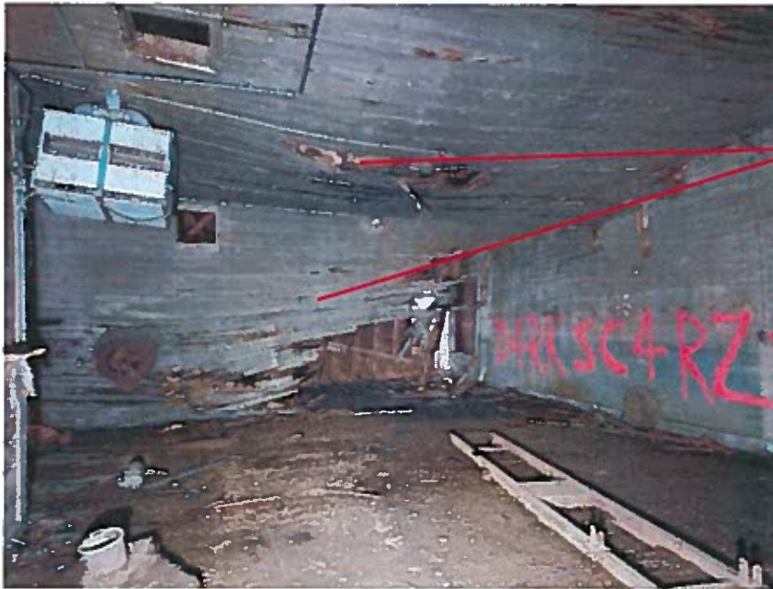
Image shows major damage to the ceiling of the structure.
