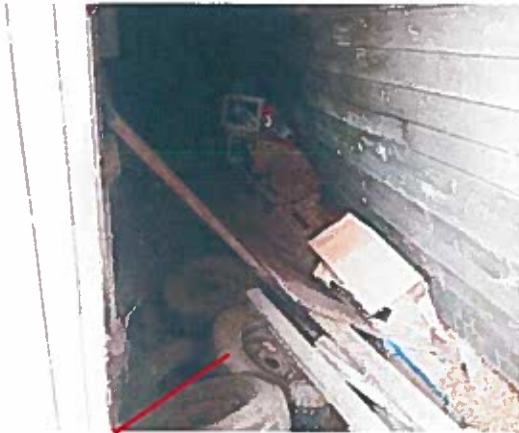
Used tyres noted in the structure.
