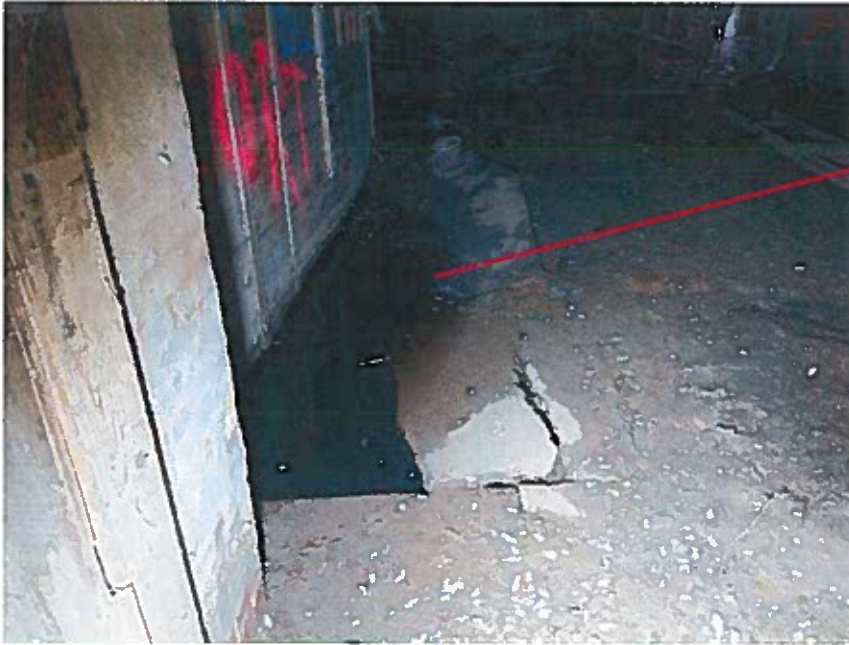
Image shows a large hole in the floor filled with water.
