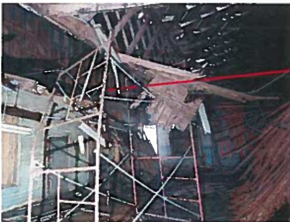
Buckled safeway style scaffolding supporting the weight of the collapsed ceiling.
