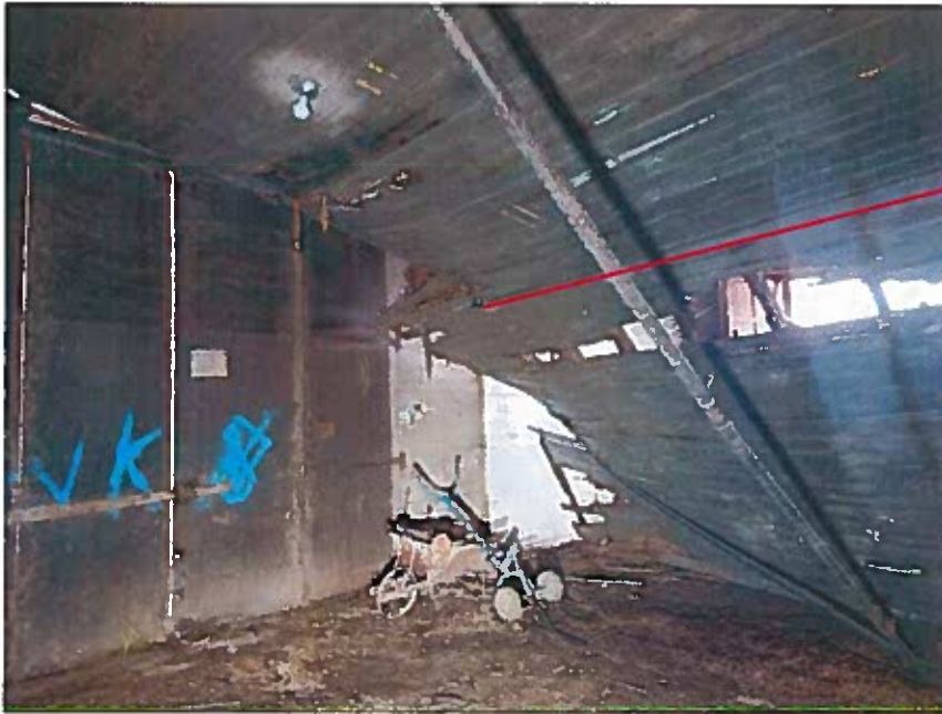
Image shows partially collapsed ceiling.
