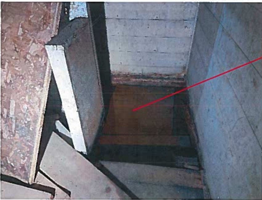
Image shows stairwell to basement completely submerged in water.
