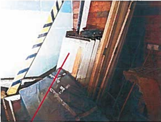
Ballasts and Fluorescent light fixtures can contain PCBs.
