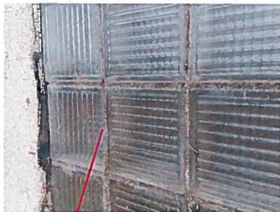
Window caulking at front of building. Chrysotile 10-20%
