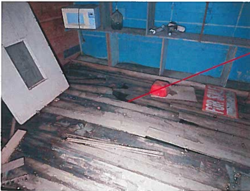
Image shows dangerous flooring with rotten floor boards.
